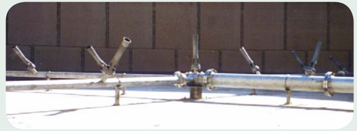
Jet Mixing System in tank
