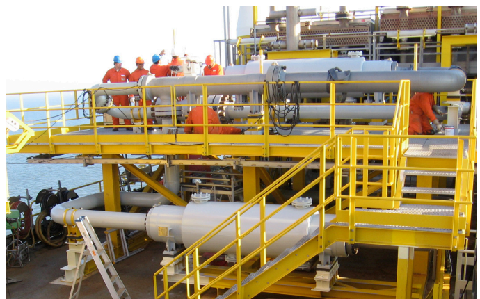
Gas Ejector complete with Silencers installed on Rig
